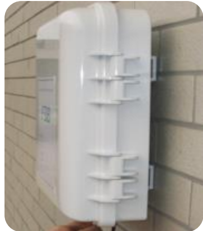
FTTH termination box in the building
